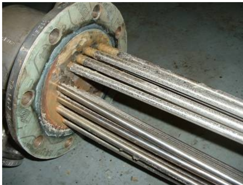
Heat exchanger aboard the Norstream, 22 nd of May 2006
