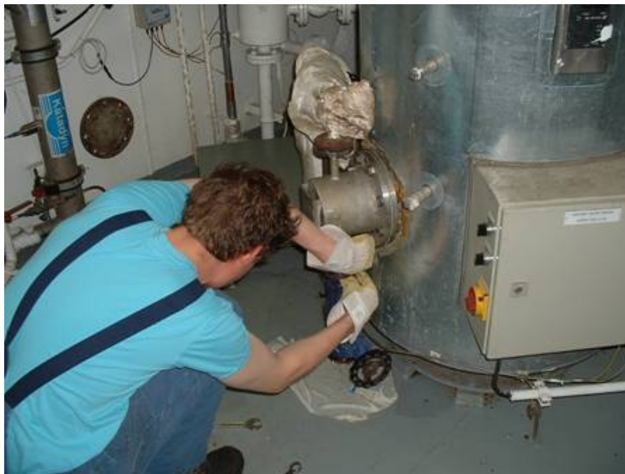
Opening of the Heat exchanger aboard the Norstream
