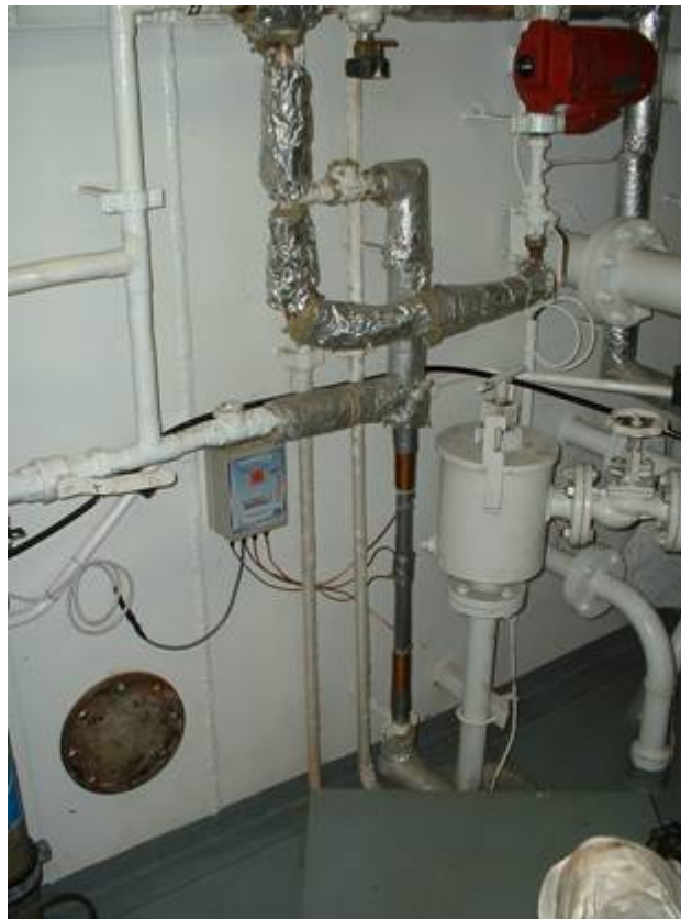
Hydrosmart installed aboard the Norstream
