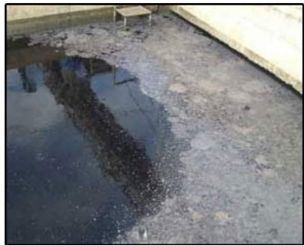
Fig. 3 Sludge in pond A
