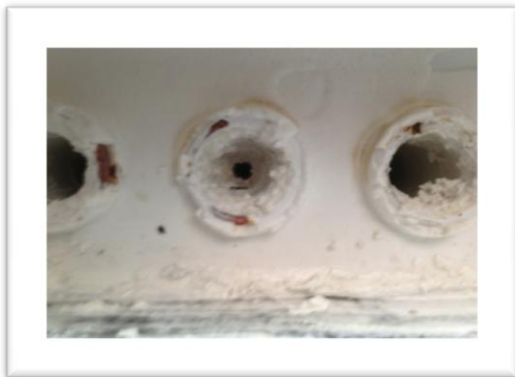
Before De-scale system installed
